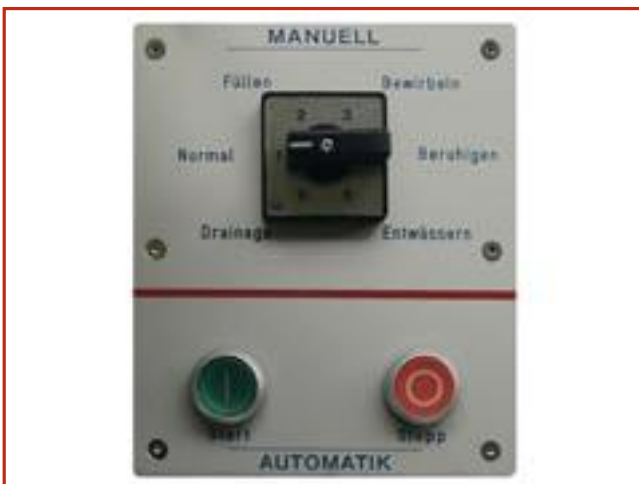
Manual and automatic control
